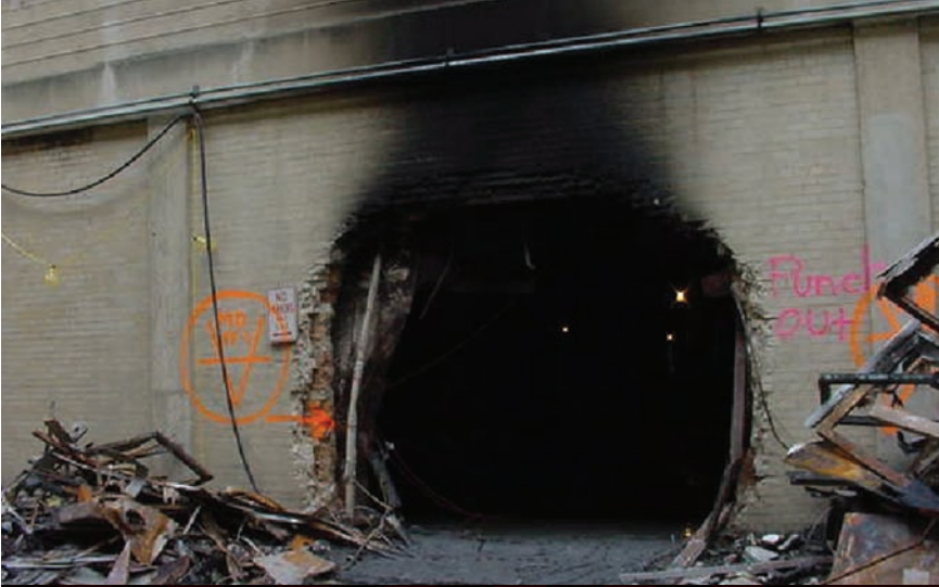
A view of the hole that Flight 77 created through the inner C-Ring wall, opening onto A-E Drive (Note the FBI markings and the designation "Punch-out [hole].")
